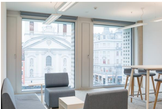
Fig. 5: MIREL evolution pendant luminaires mounted above the computer workstations in the post office headquarters ensure optimal visual comfort. As a special feature of the lighting concept, these fittings are equipped with two different light colours: 4000 K direct light and 3500 K indirect light.
